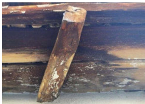
Figure 4b Hyphodontia crustosa on roof construction of Monastery guest house.
