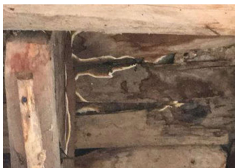
Figure 5 Coniophora puteana on roof construction.
